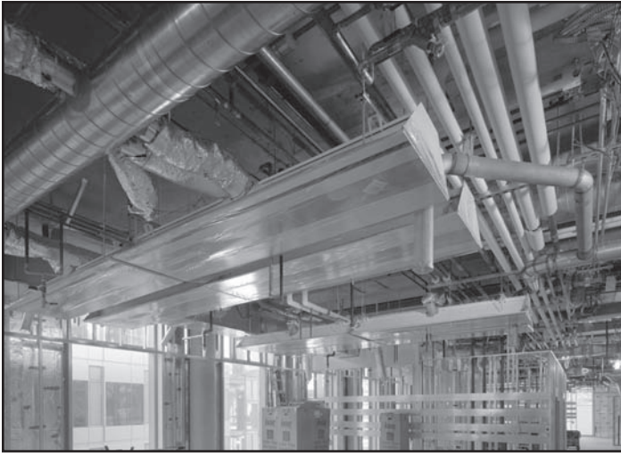
FIGURE 2: Active chilled beam installation. Note smaller-sized conduits. (Photo courtesy of John Edwards.)
