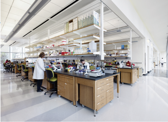
The flexible laboratories allow research group sizes to expand into adjacent neighborhoods. Chilled beams, located about the benches, reduce heat gains from instruments and equipment on the benchtops. Photo: Eric Staudenmaier
